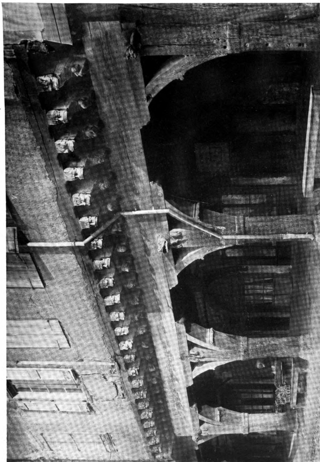
Woodwork—Mirepoix (Ariège) Galerie de la Place—Showing carved beam ends as found in stonework
